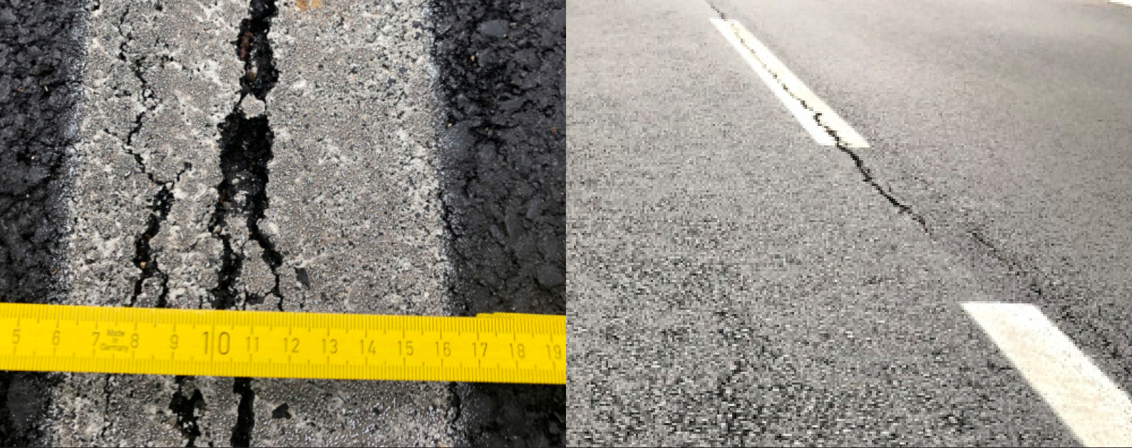
The road condition prior to application of the Tensar solution.
