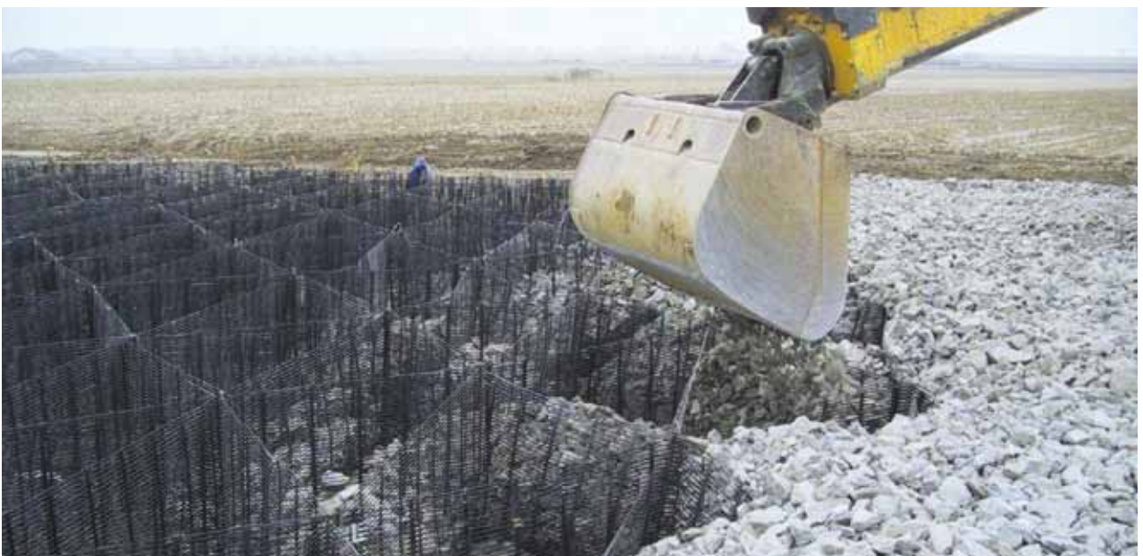
3. Approved fill is carefully machine placed into the cells and requires no compaction.
