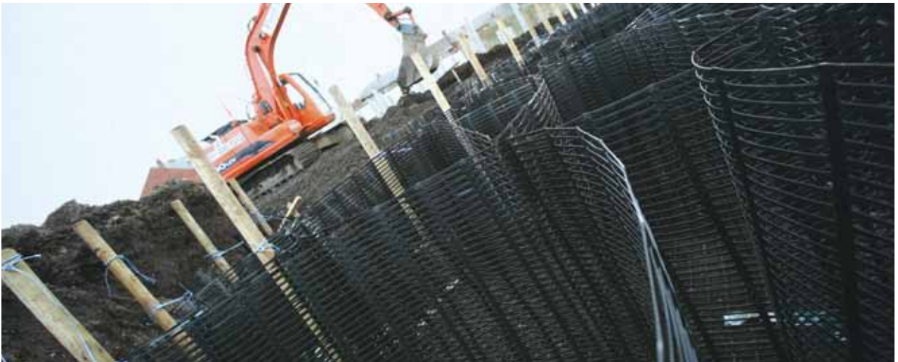
Proven application of the TensorTech® Stratum™ System for construction of an access road over very soft and wet ground conditions (Northumberland, UK).
