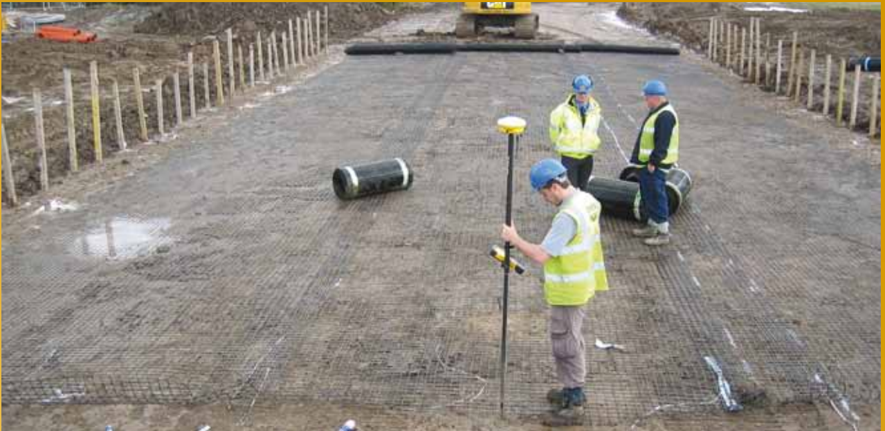
1. The base of the cellular foundation mattress system is quickly formed by unrolling geogrids onto the formation.
